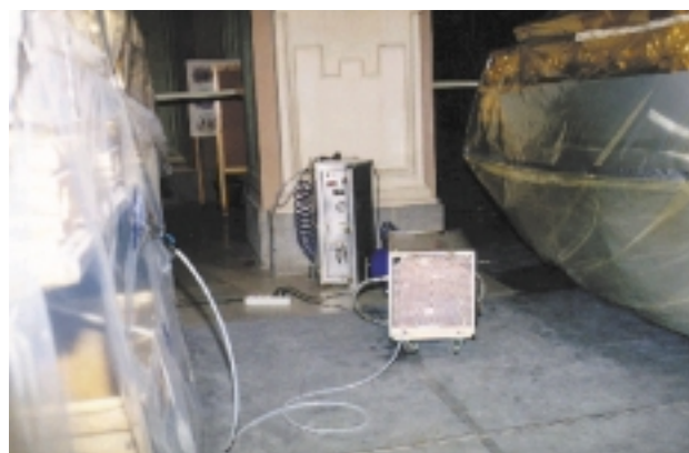
Figure 2. Velox equipment maintaining a nitrogen flow in the enclosure.
